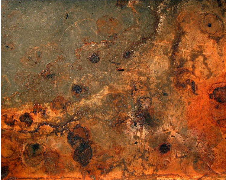
Fig. 15. Rust-The most familiar example of corrosion
