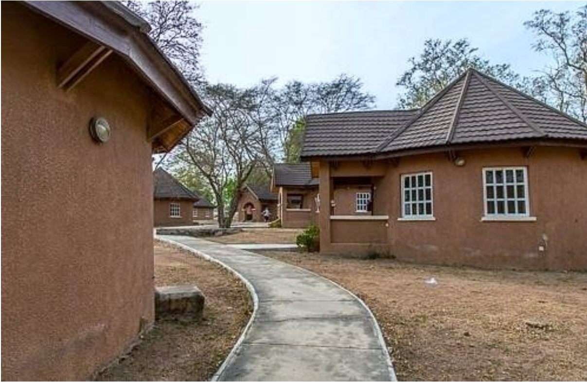
Figure 42: Dilapidated visitor accommodation at Yankari Game Reserve reflecting poor maintenance and urgent need for facility upgrades.
